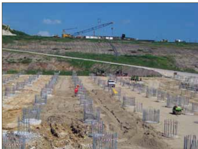
Changi treatment facility, Singapore.
