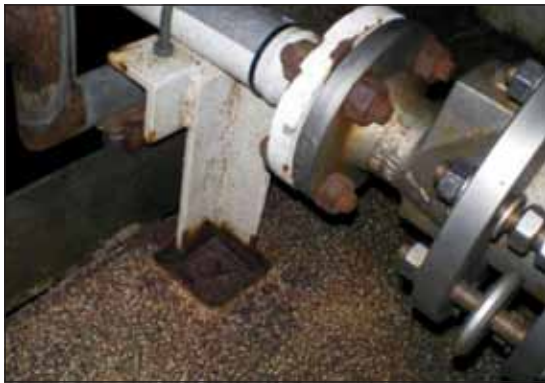
Figure 22: Failing carbon steel bolts in stainless flanges.
