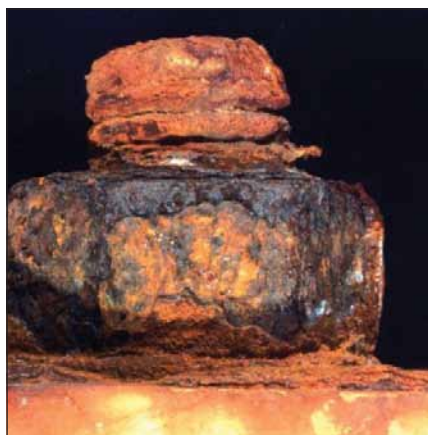
Figure 2: Rusting bolt from DNV testing.
