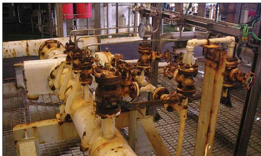
Figure 1: Rusty valve deck on offshore infrastructure.
