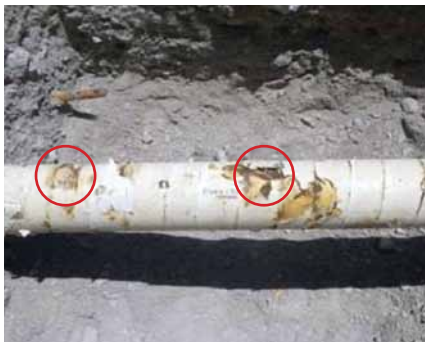
Damaged outer wrap caused by the backfill.
