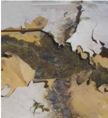
Notice the damage to the outer wrap. The outer wrap has "sacrificed" its protective layer. The outer wrap was removed to reveal a perfect, intact and undamaged DENSO petrolatum inner wrap.
