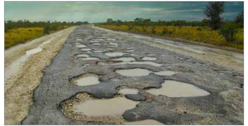
South Africa now has more potholes than households. Photo credit: https://mybroadband.co.za/
