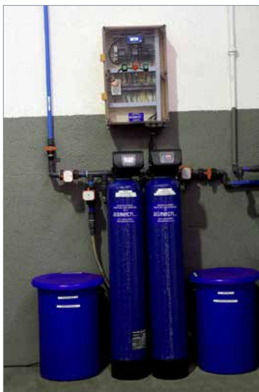
Allmech's demineralisation plant.
